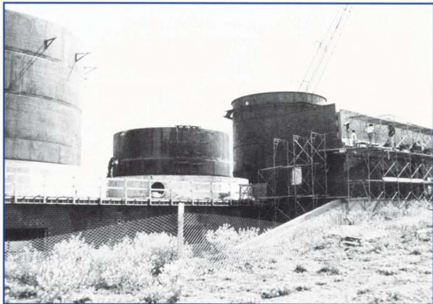
THE SMALL WHITE AREA SLIGHTLY left and down from the workers on the building (in the right of the photograph) is the opening through which the Serpentix conveyor from the dewatering building will enter the composting plant (also see artist's rendering on Page 8).
