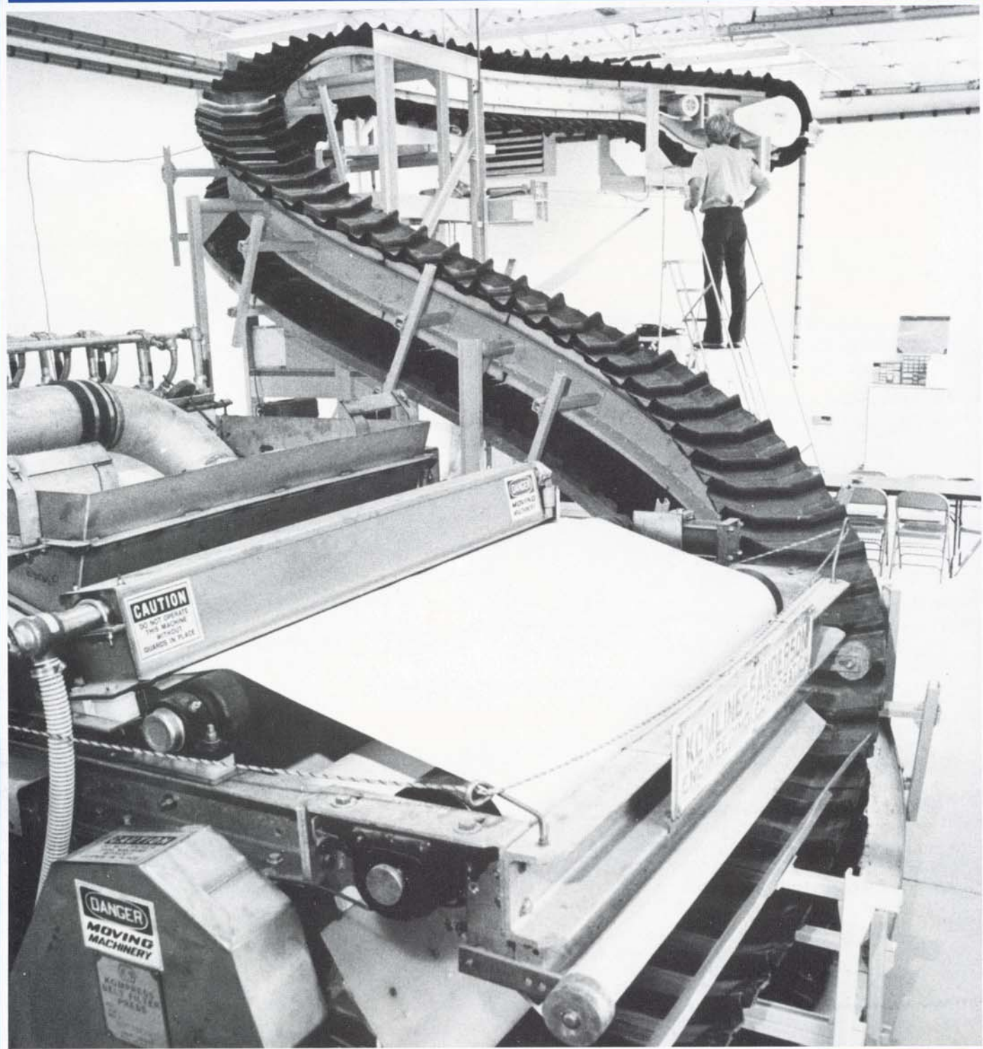
Sludge Cake Discharges Over 12 Foot Arc
