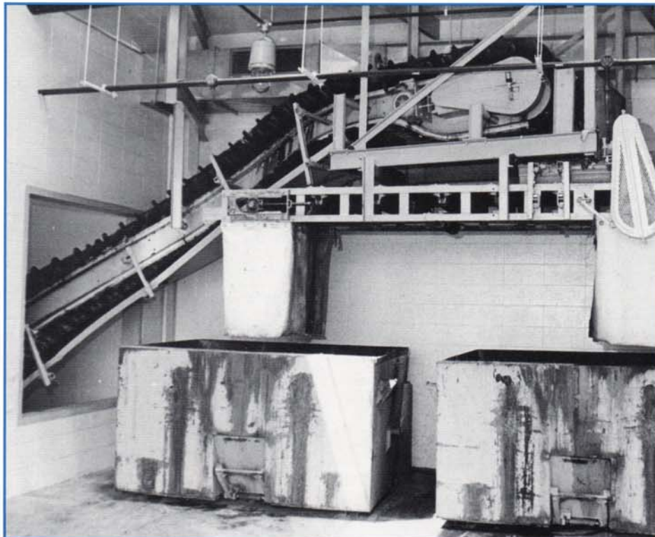
AT THE END OF ITS U-SHAPE, the screenings conveyor (lower left photo) makes its third 90-degree turn to the left, followed by the 105-degree helical turn to the right. IN TOP RIGHT PHOTO the conveyor is seen passing through an opening in the wall, completing a 32-degree incline, and discharging from 10 feet above floor level onto a flat belt shuttle conveyor for discharge into dumpsters.
